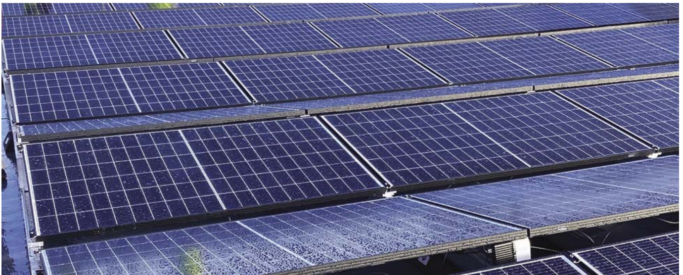
Solar panels have been installed on the roof of Eckington Swimming Pool and Fitness Centre
